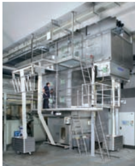
EcoFix®/2 heat-setting plant at a German customer's location
